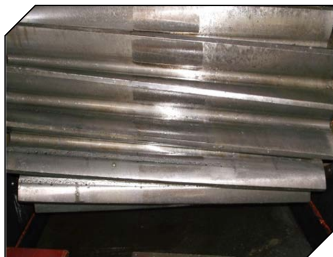
Figure 1 Example of girth gear misalignment: girth gear driving pinion end is aligned to the reducer, causing misalignment between the girth gear teeth and driving pinion teeth (courtesy HMC).
